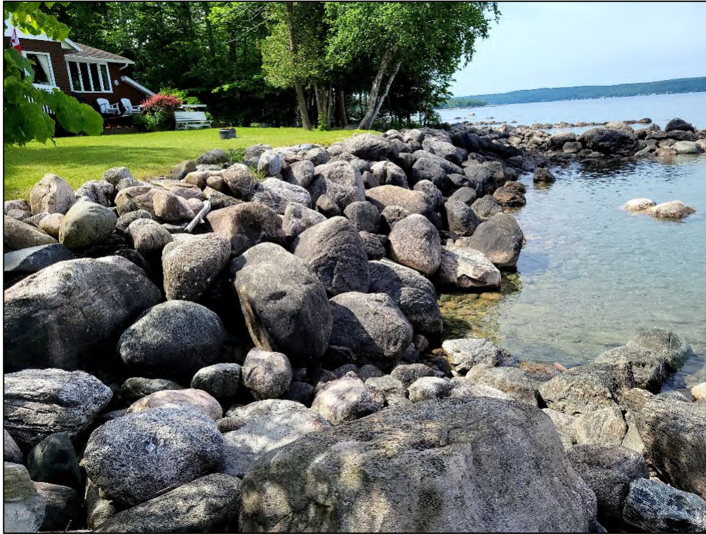
Photo 1 Existing Revetment at Property 0283, June 2025
