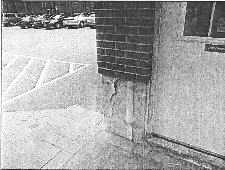
Photo 6 – Corner Spalling on Southeast Corner on Addition Foundation
