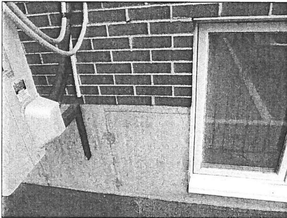
Photo 7 – Minor Cracking Beside One Basement Window on North side of Addition
