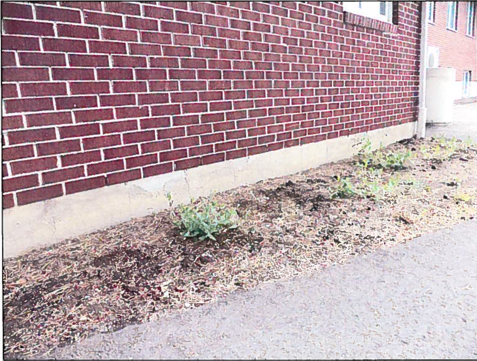
Photo 9 – Cracking at Top Course Head Joints of Concrete Block Foundation, Entrance Lobby at Northeast Corner of Addition
