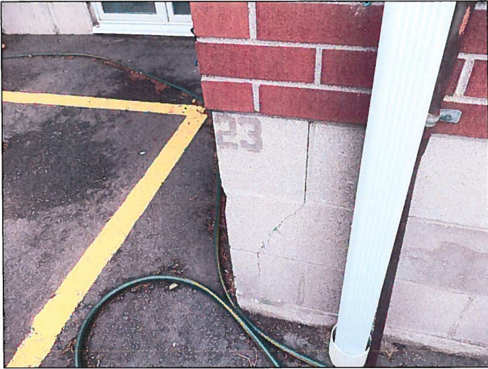
Photo 5 – Corner Spalling at Foundation of the Original Building
