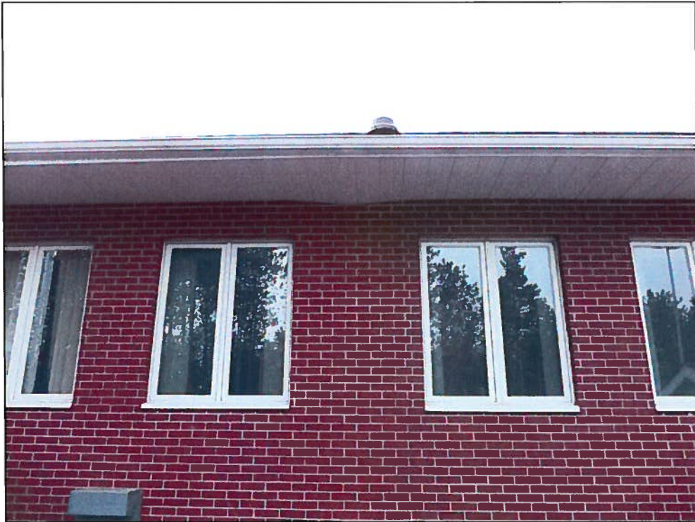
Photo 10 – Three Foot Section of Damages Soffit at South Side of the Addition
