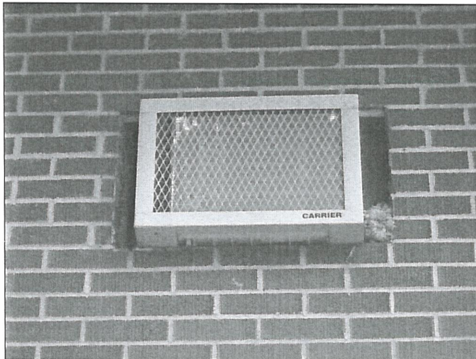
Photo 8 – Oversized Opening at Ground Floor AC Near Northeast Corner of Addition
