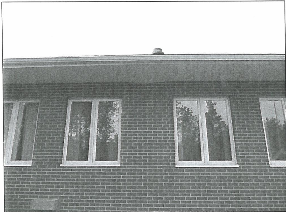
Photo 10 – Three Foot Section of Damages Soffit at South Side of the Addition
