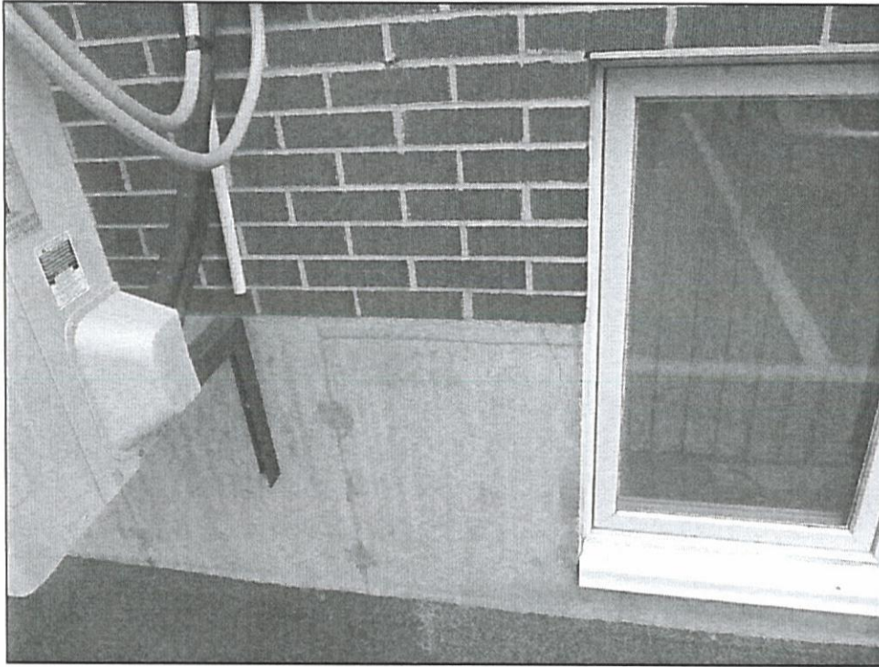
Photo 7 – Minor Cracking Beside One Basement Window on North side of Addition
