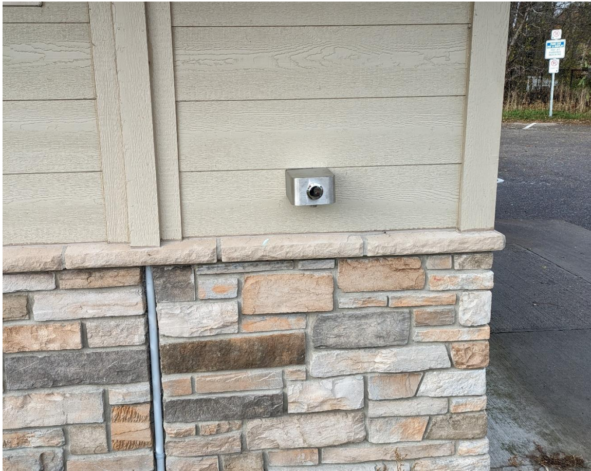
Image of one of the water fill stations.
